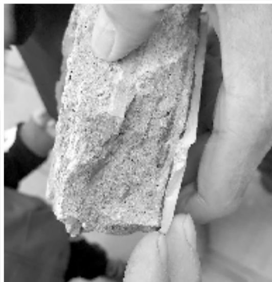
莱茵园外立面掉落的砖
